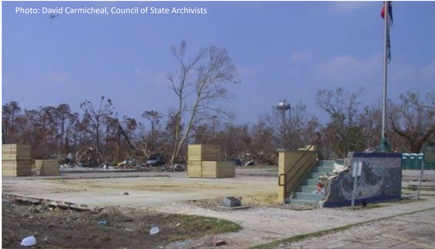
Waveland, MS City Hall after Hurricane Katrina
