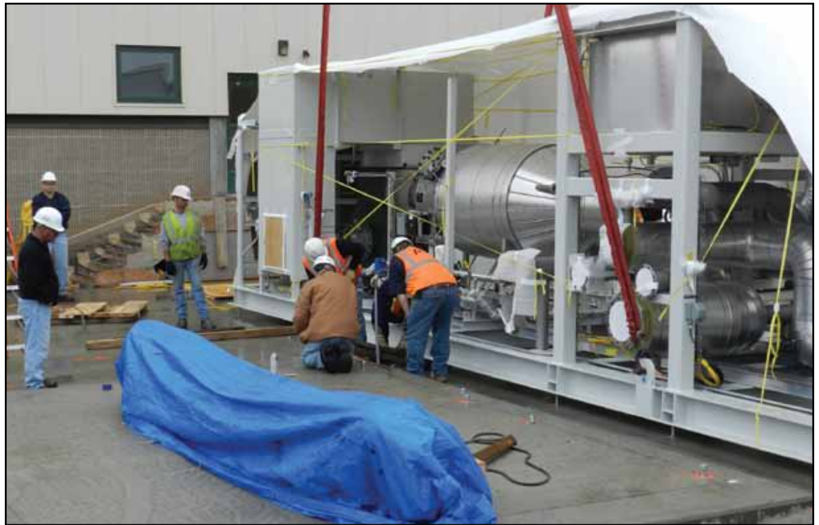
Components of Greenwood Energy's Direct FuelCell® power plant are assembled next to East Hall as CCSU becomes the first university in New England to use the "green" technology to generate power for a large portion of its campus.
